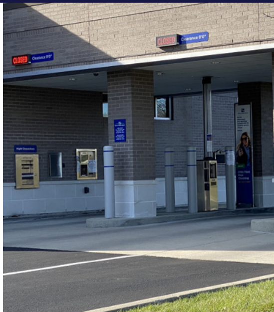
Interactive Teller installed in Lane 1
